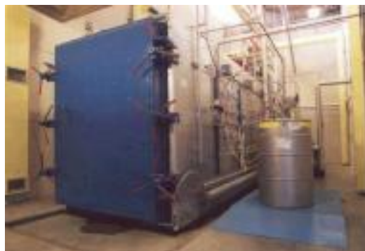
Figure 15: Ethylene Oxide (ETO) sterilization plant.
